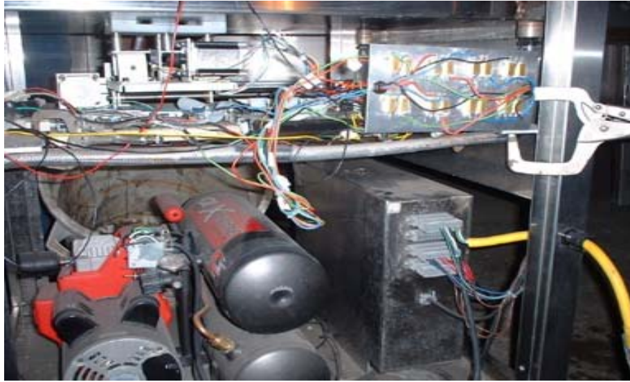
Fig. # 9: High Pressure Injection Cabinet System
